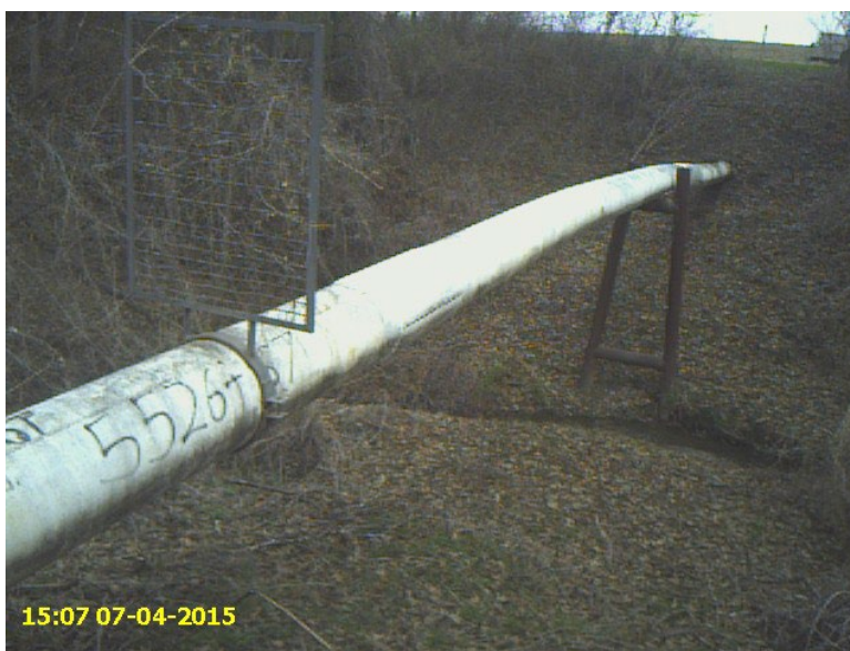
Photograph 2: Photograph of Span 6-5526+67-5260 in Buchanan County, MO, taken on April 7, 2015, showing no sign of staining.
