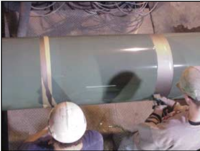
Removal of tape from shop system to expose area for simulated girth welds.
