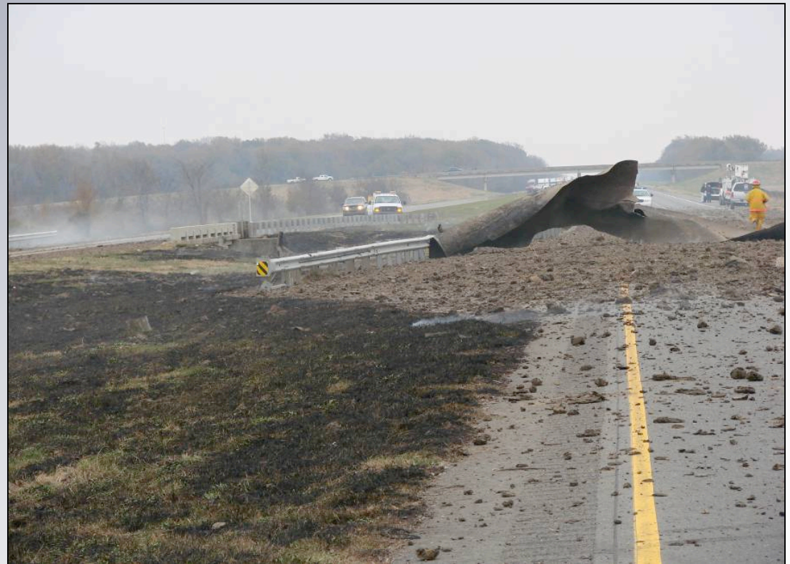
Failure of Cased Crossing Under Highway
