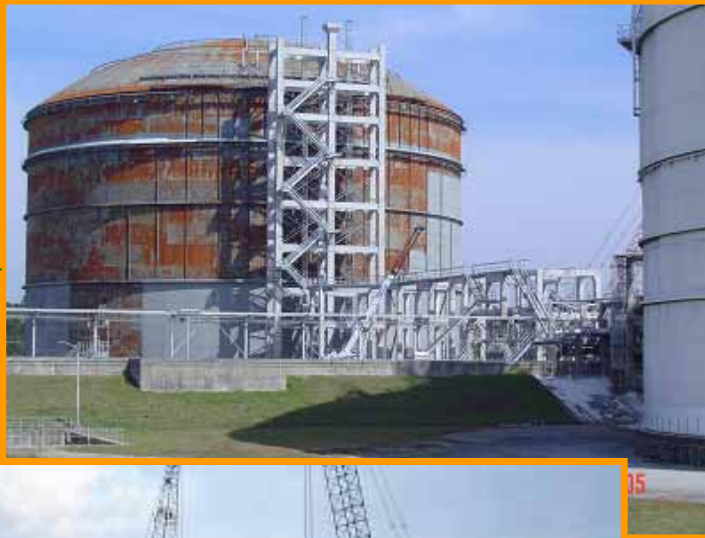
Tank D & Trestle
