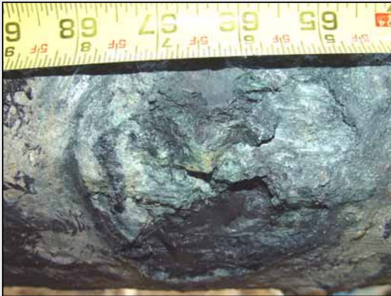
Salt deposit and coating defect
