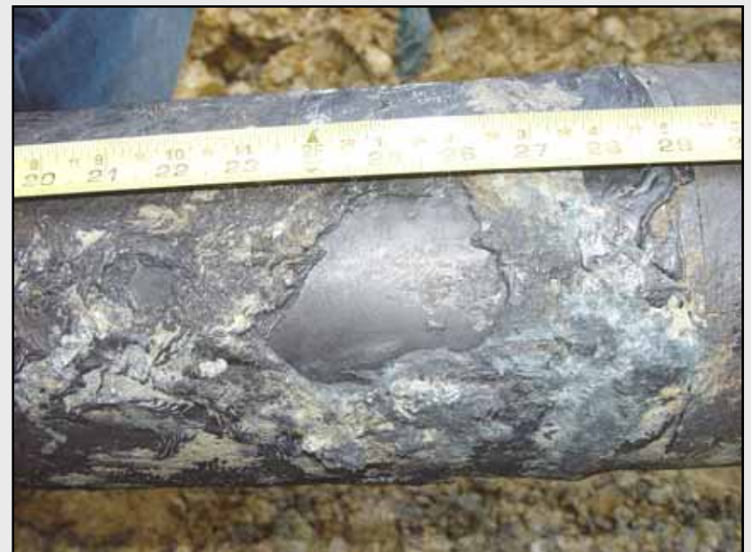
Large coating defect
