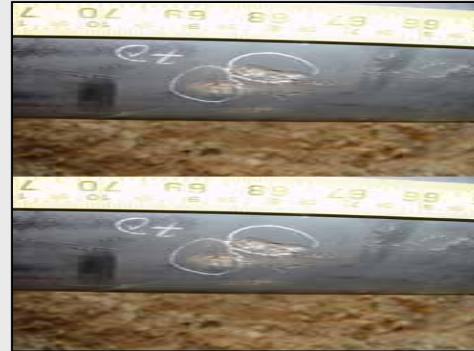
Corrosion defect on bottom portion of pipe
