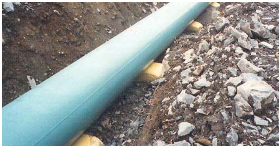
Figure 5.6 – Pipeline on Foam Supports ( http://www.pedero.com )
