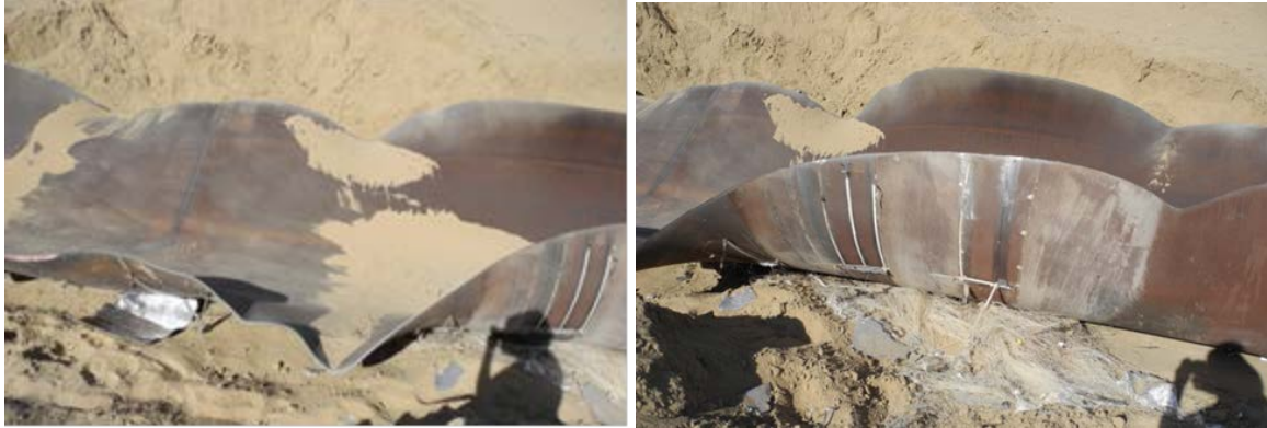
Figure 16 Damaged pipe at the center location and towards Pipe #753 end
