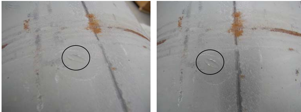
Figure 69. Area of mechanical damage on the external section of a pipe section.
