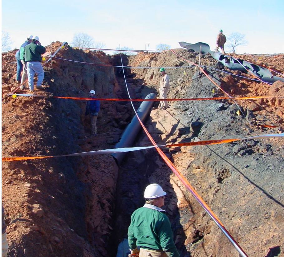
a) view uphill toward the location of the failed wrinklebend
