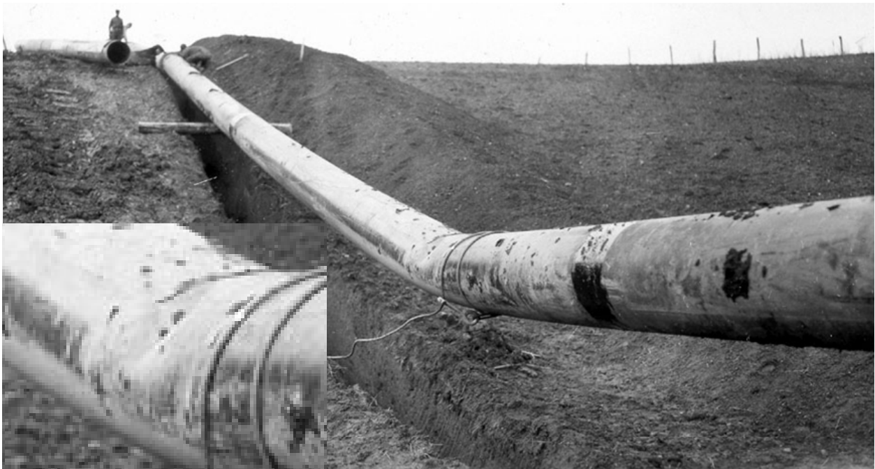
Figure A2. Wrinkle made hot over a machined ditch by dead-weight sag method – inset view shows some significant local distortion develops in the cross-section (circa 1930s)
