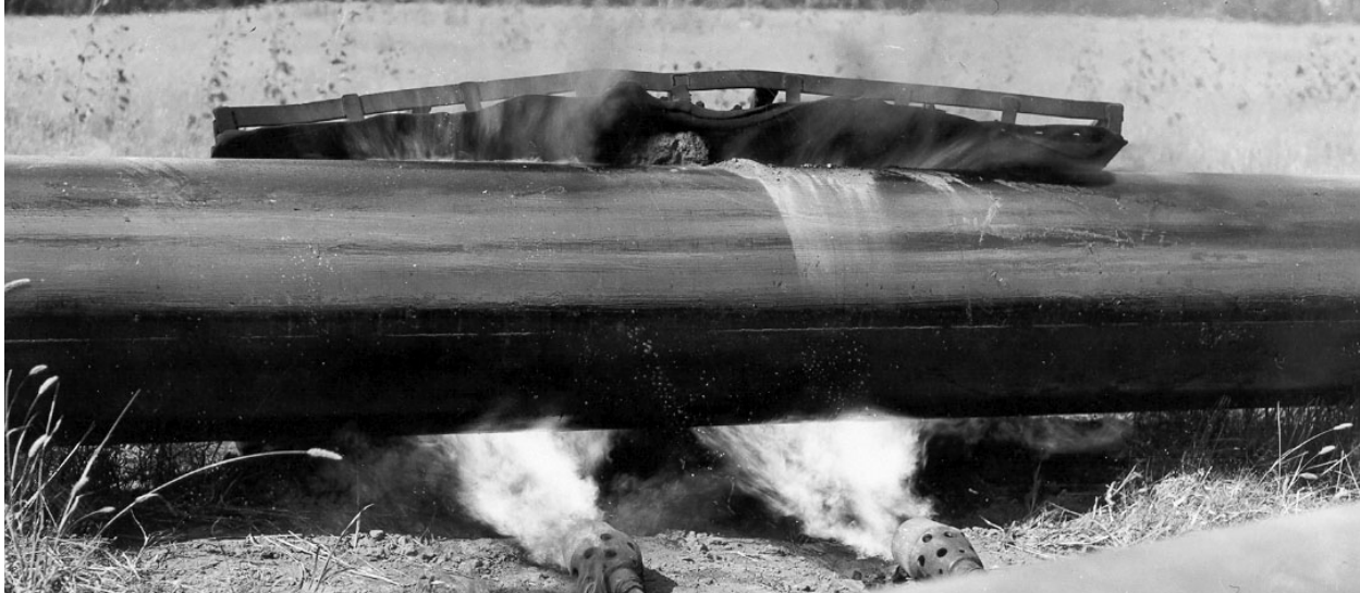
Figure A5. Heat being applied via oil burners for hot wrinkle-bending, with a fixture to distribute the heat (1930s).
