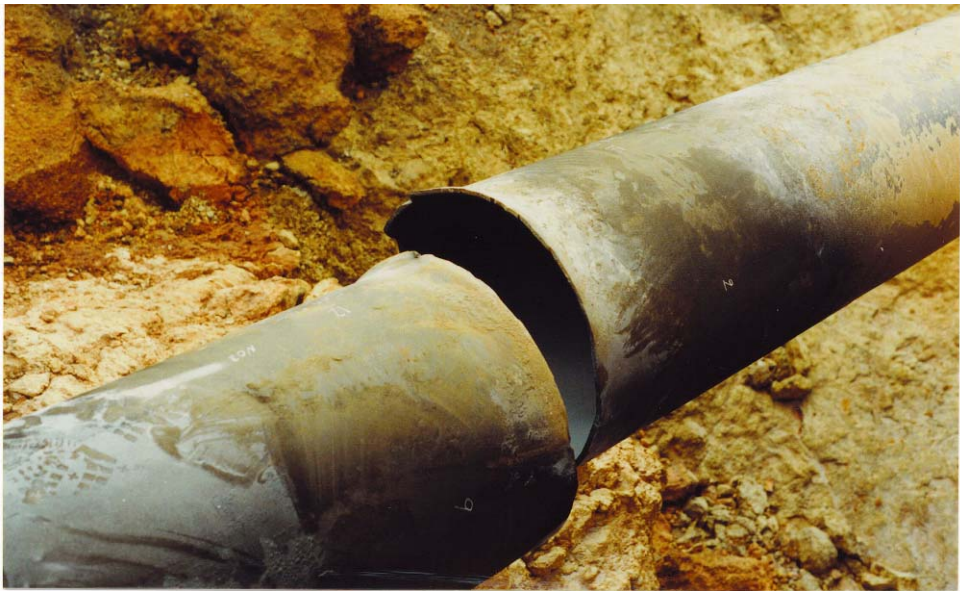
a) overview of failure
