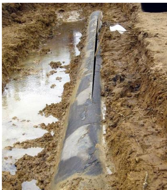
Figure 10 Brittle fracture of vintage (1948) pipeline along an ERW seam weld
