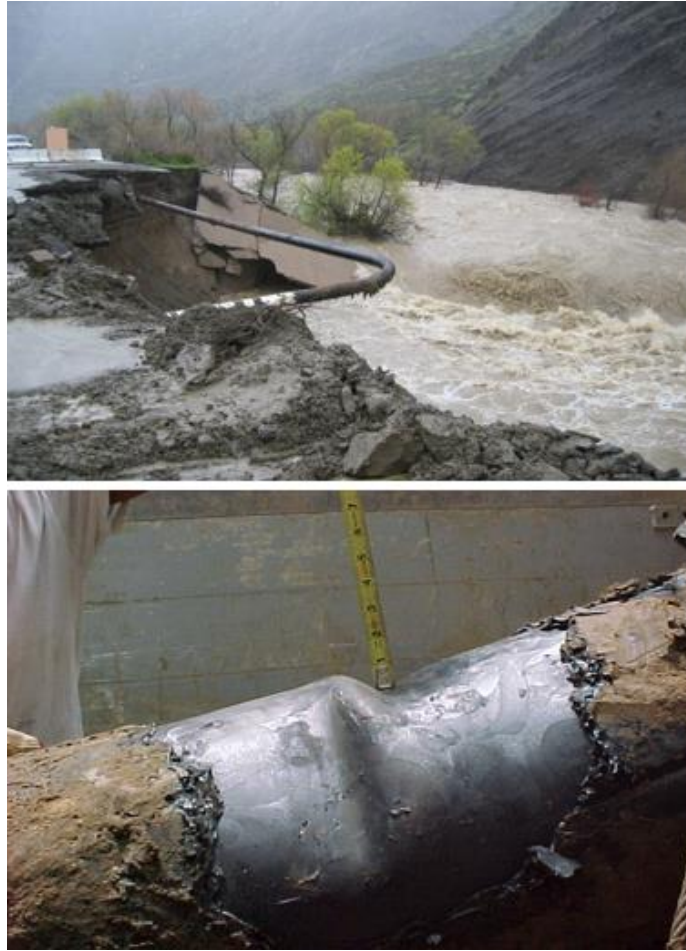
Figure 42 Illustrations of natural force damage to a pipeline
