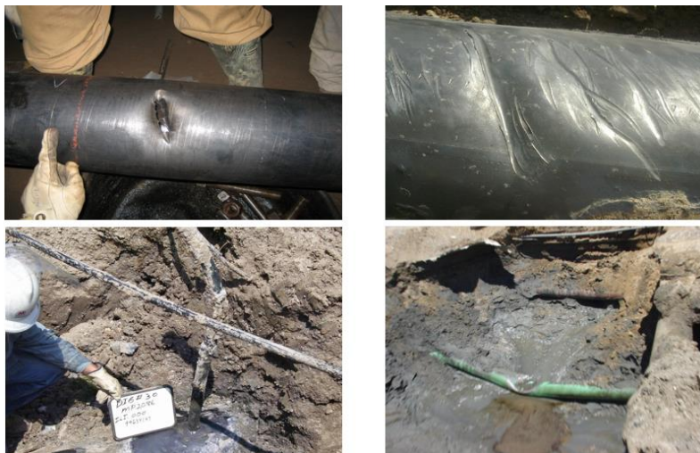
Figure 35 Illustration of third-party damage to pipelines
