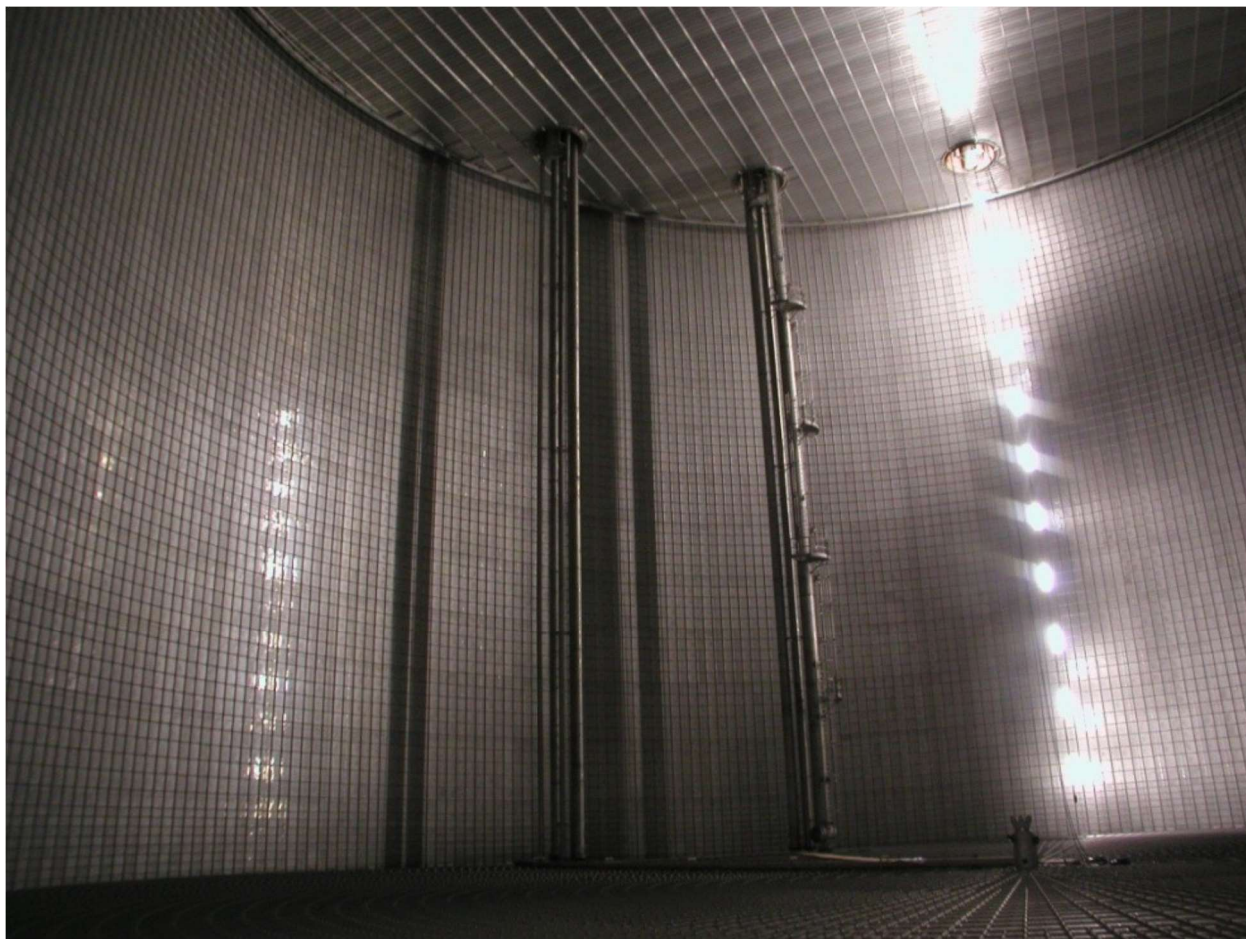
Figure 3 View of Membrane Tank Interior. The liner is stainless steel with membrane corrugations forming a square pattern.
