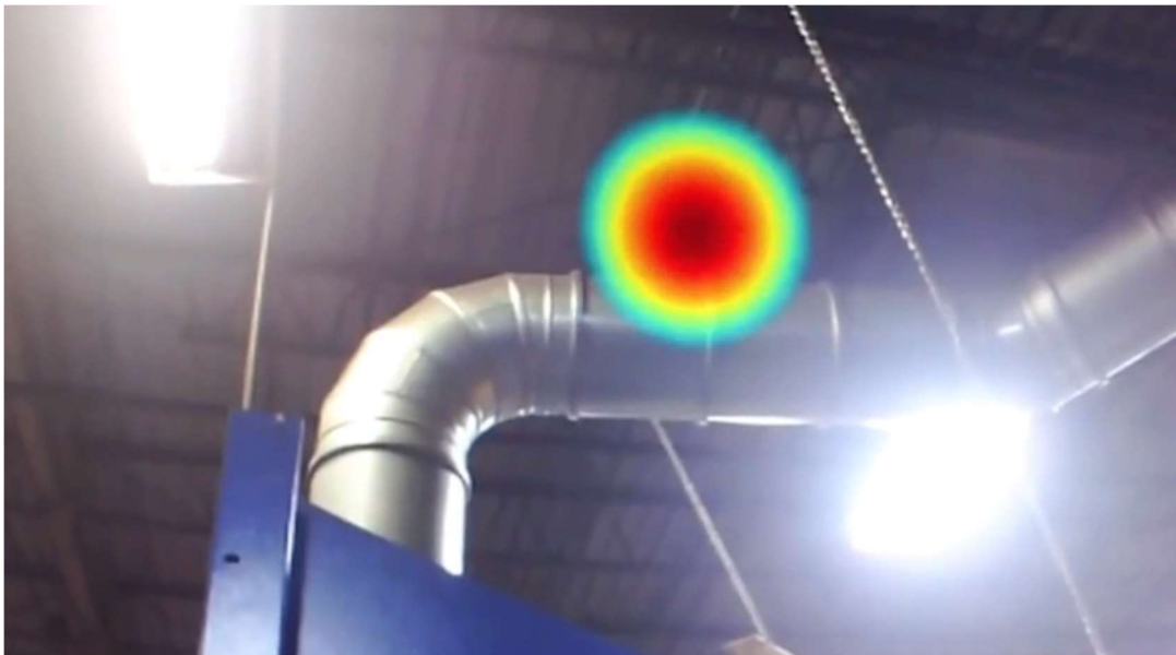
Figure 11 Acoustic Imaging Showing Leak Location
